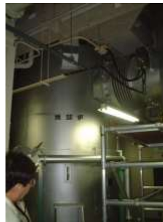
Feeding to incinerator ( self-sustained combustion type)
