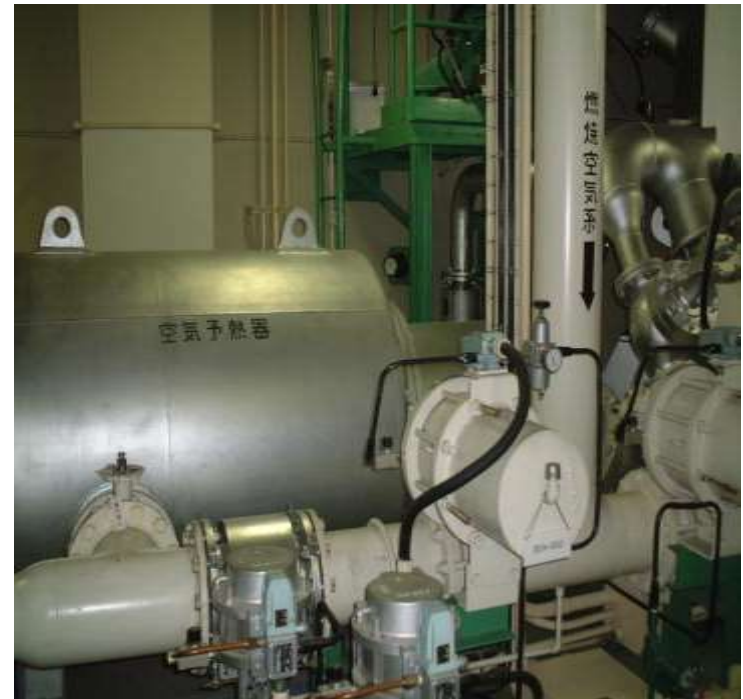
Air pre-heater (incineration mixed with propane gas)
